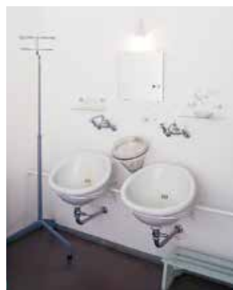
廊下側 手洗い器
